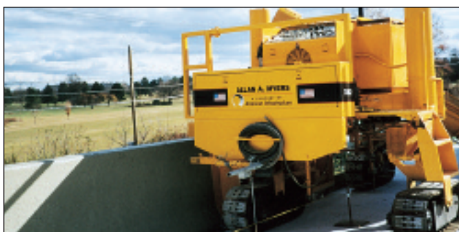
No problems or leaks were found during reconditioning of the 5700 for bridge work
