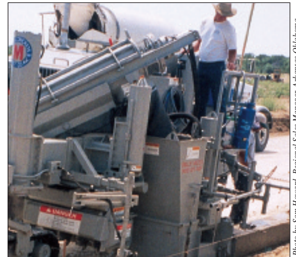
The SUPER-B has made life easier for the Moss Concrete crew, with the guys doing very little touch-up work, says Billy Moss
