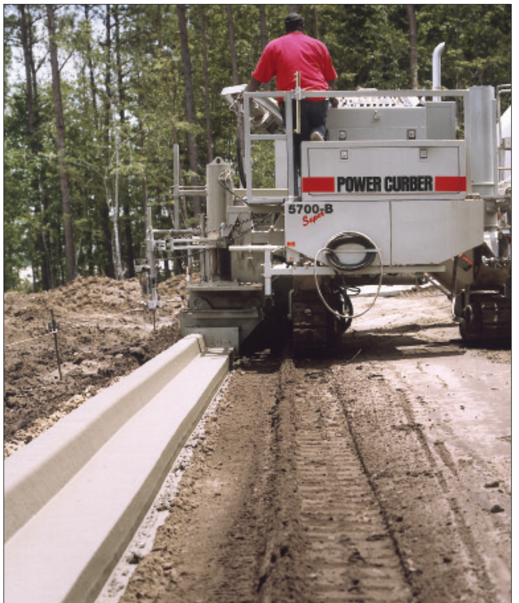
The SUPER-B 's compactness makes moving the machine from job to job throughout South Carolina and Georgia easy, says Malphrus Construction crew
