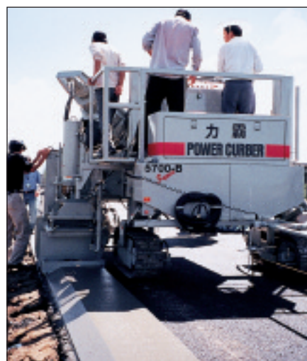
This road edging is being slipformed by the Inner Mongolia New Development Road & Bridge Construction Technology Co.
