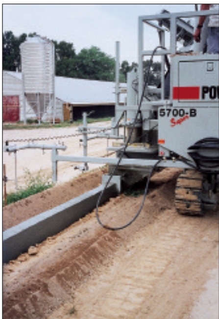
The footer is slipformed in the trench dug by a wheel in the center of the special trimmer
