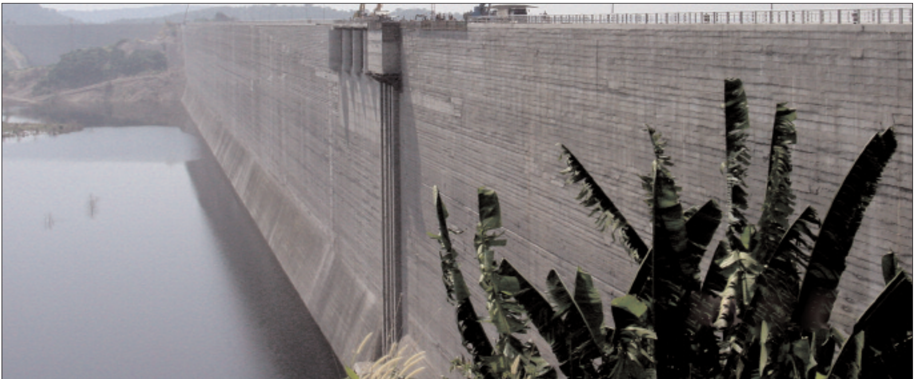
Four Power Curber machines slipformed more than 1.7 million feet of concrete in the two faces of the dam in Thailand
