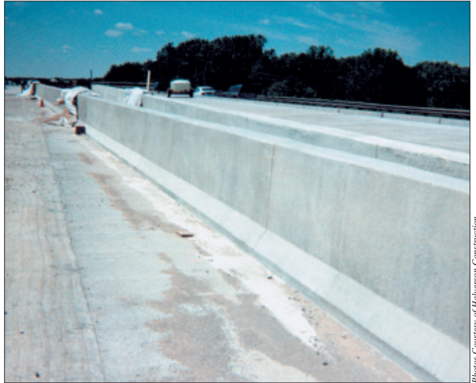
With the 5700-B on the road so much pouring parapet as well as curb and gutter, reliability is a key, says Kelvin Long, machine operator
