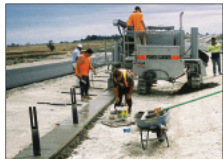
Crew knocks posts into concrete-filled bore holes in the concrete strip. The strip is being slipformed by the SUPER-B. The new post hole digger attachment allows the SUPER-B to dig the holes in the same pass as the machine trims the sub-grade
