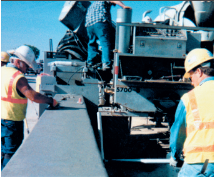
In this pour on an Interstate 57 over Route 40 in Effingham, IL, the barrier is 19 inches wide (48 cm) at the top
