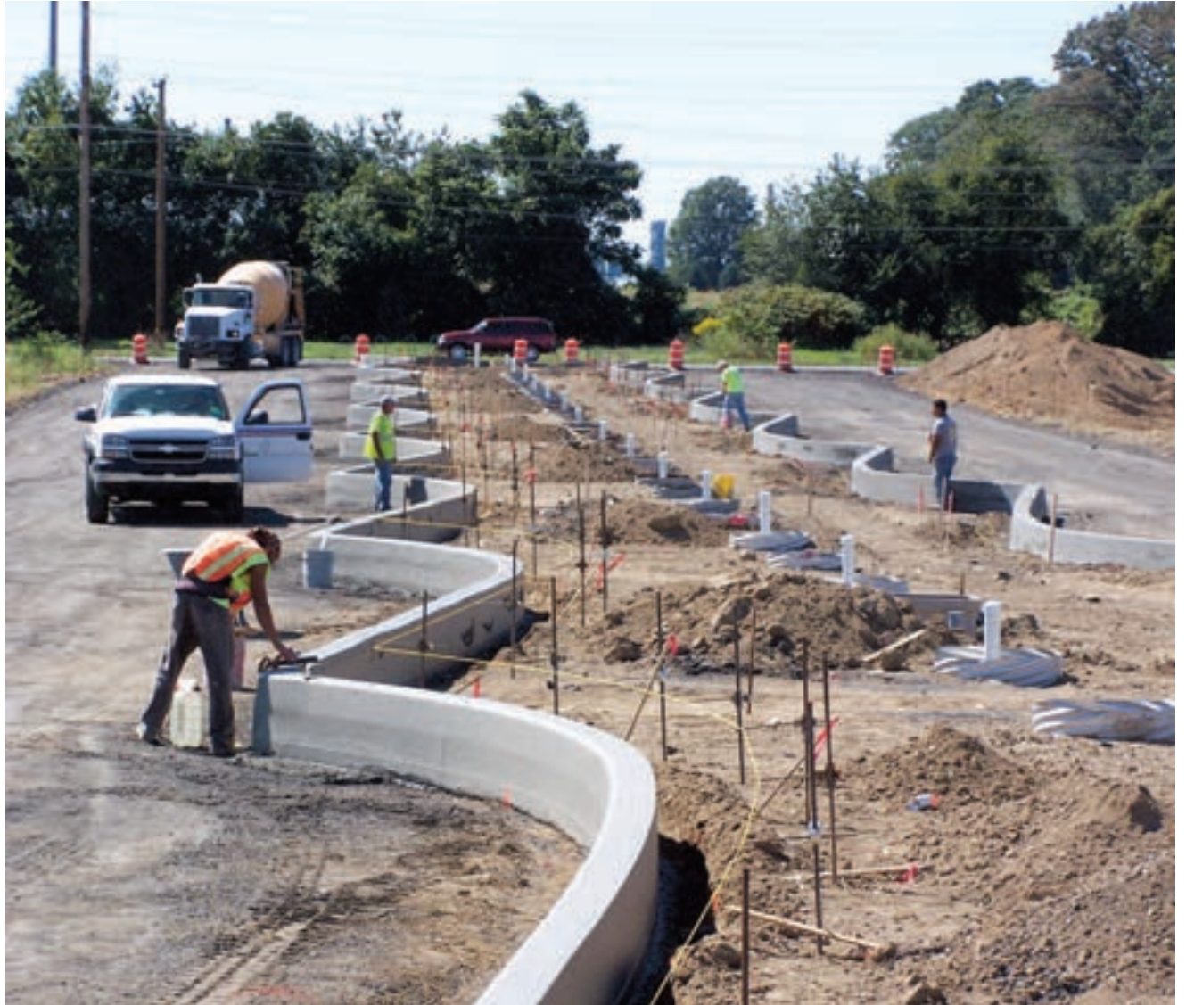
Multiple radii poured with 5700-C on bus terminal job site in Dover, DE.
