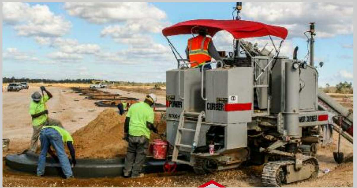
A row of freshly completed radius islands stretches into the distance as Cunningham DeLaney's 5700-C pours using Topcon Millimeter GPS controls. Photo by Dane Peters, Topcon
