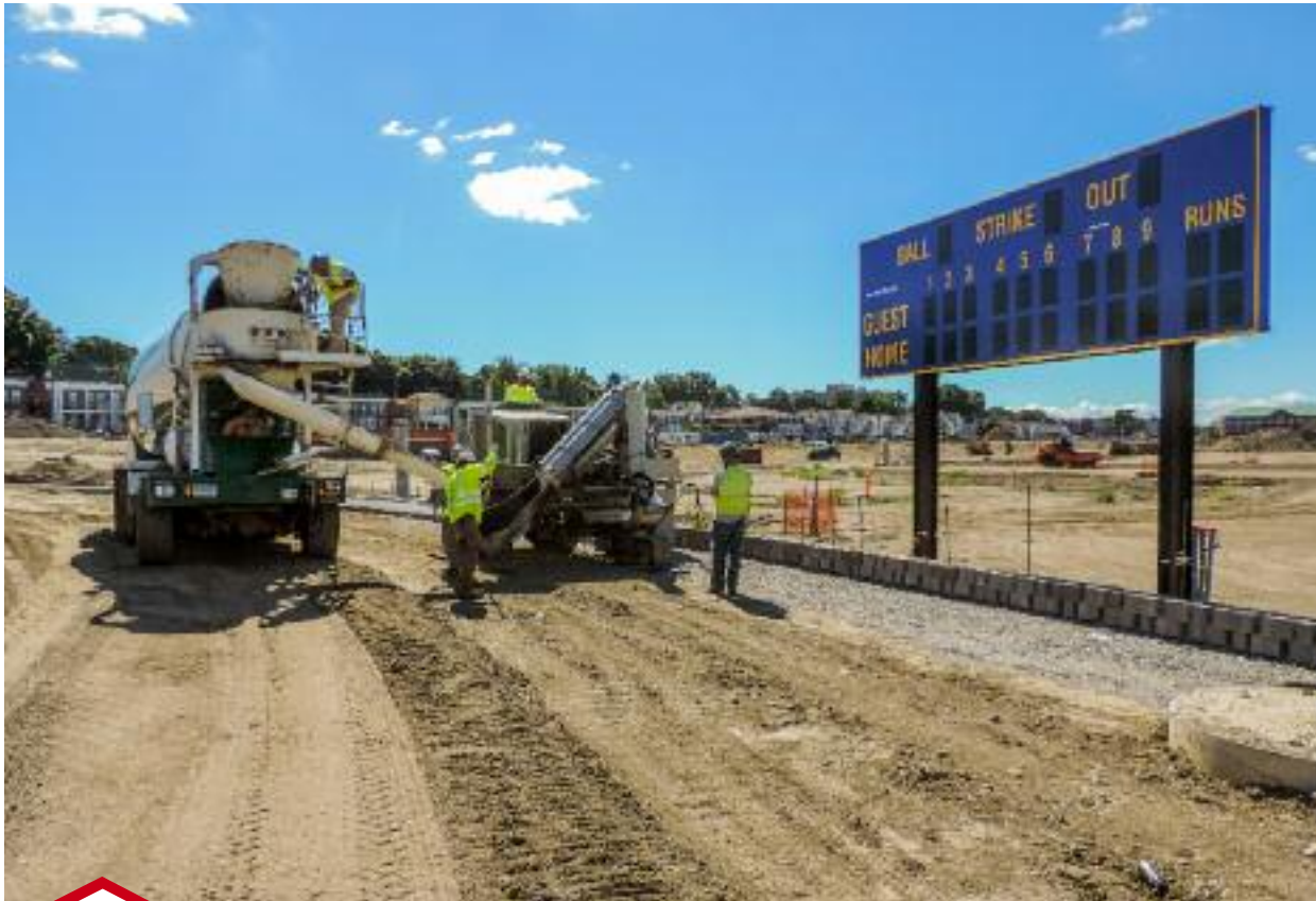
The concrete footing poured around the perimeter of the outfield will have the outfield fence posts anchored into it.
