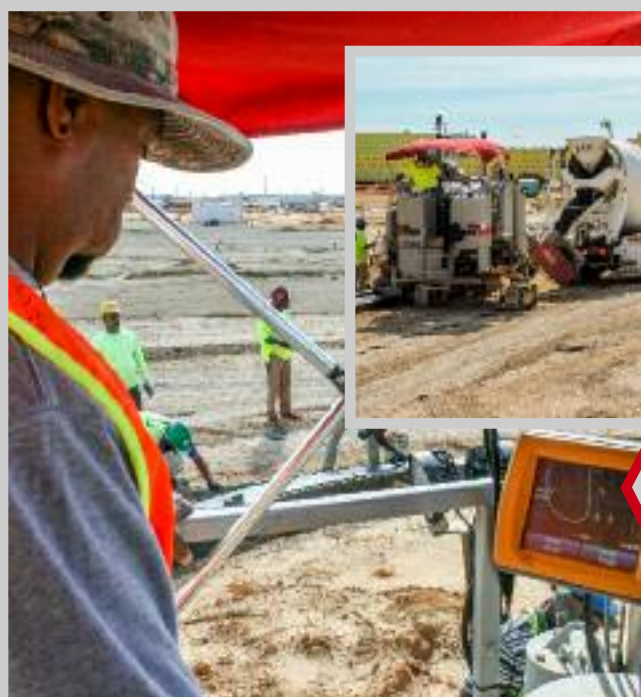
Cunningham DeLaney pours all of their sidewalk and curb with no stringline, using Topcon's Millimeter GPS machine controls. The shape of the parking lot islands they poured on this job can be seen on the Topcon display. Photo by Larry Trojak, Trojak Communications
