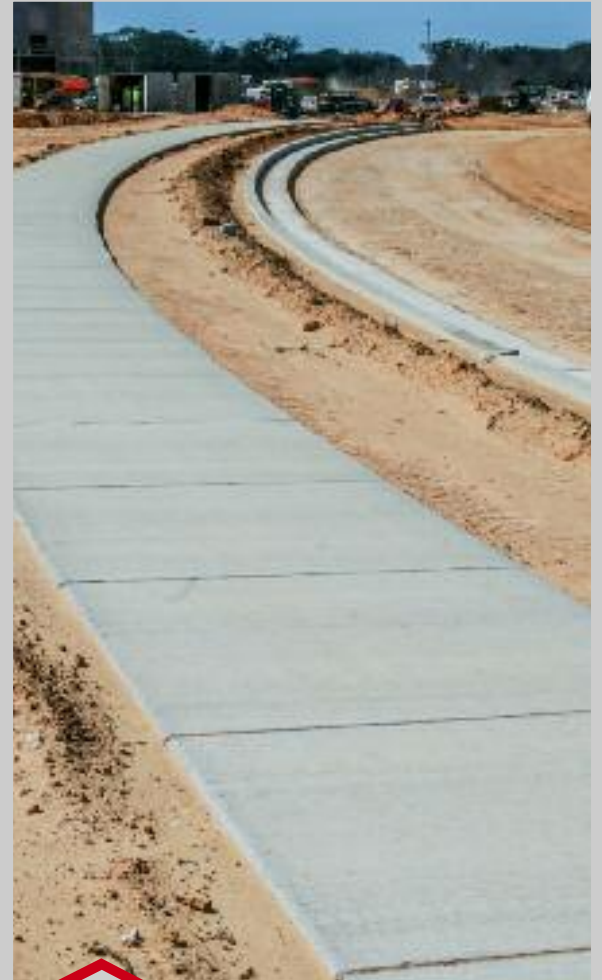
Cunningham DeLaney also poured 25,000 linear feet (7,260 m) of 5-foot (1.5 m) wide sidewalk and 55,000 linear feet (16,764 m) of curb and gutter. Photo by Larry Trojak, Trojak Communications
